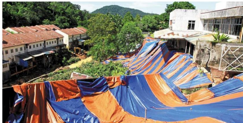
Tarpaulin sheets placed over the exposed area in Kemensah Heights, Ampang as a temporary measure following the landslide. — CHAN TAK KONG/The Star
